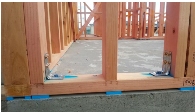
Bracing element showing “Proprietary” hold down bolt/bracket.
